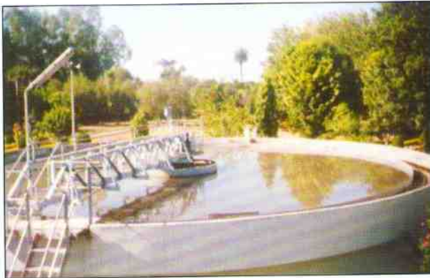
UASB Sewage Treatment Plant at Kankhal (Hardwar)
