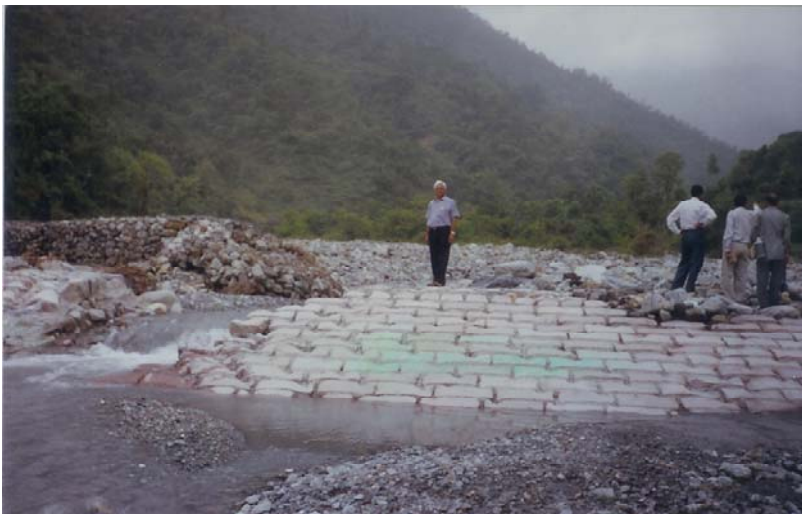
Figure 2: Breach in Kota Weir (Photograph taken in year 2002).
