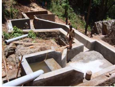
Fore bay tank.
