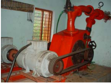
Pelton turbine and alternator.
