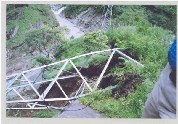
Damaged Transmission line of Urgan (3000 kW) SHP
