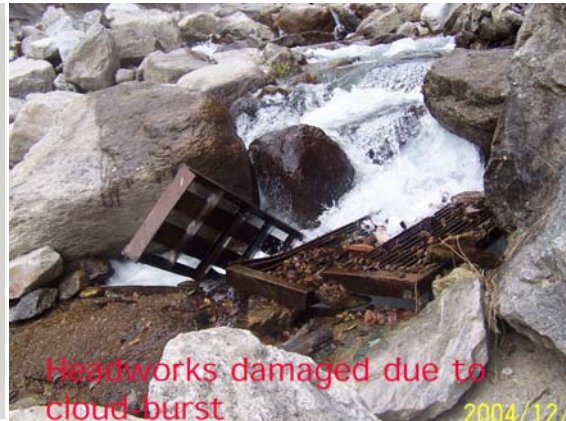
Damaged Headwork of Chirkilla (1200 kW) SHP
