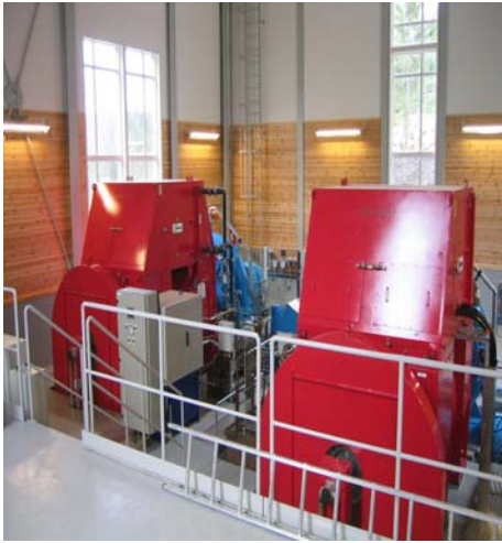
Uleberg machinery room
