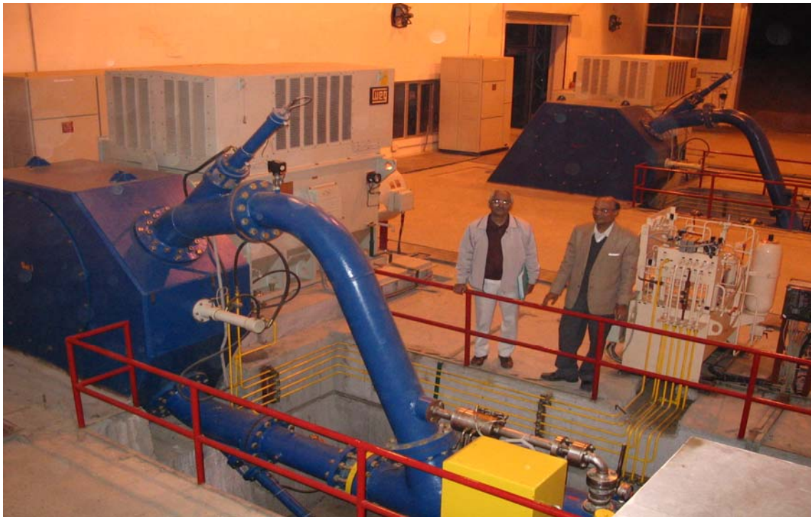
Aleo HEP Generating equipment
