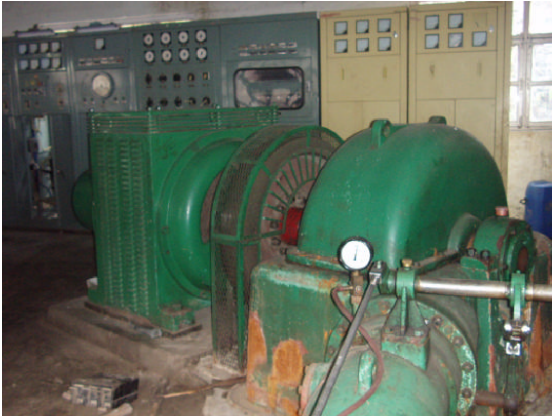
Fig 2: One of the 250 kW unit of a 2 MW SHP plant in Western Nepal
